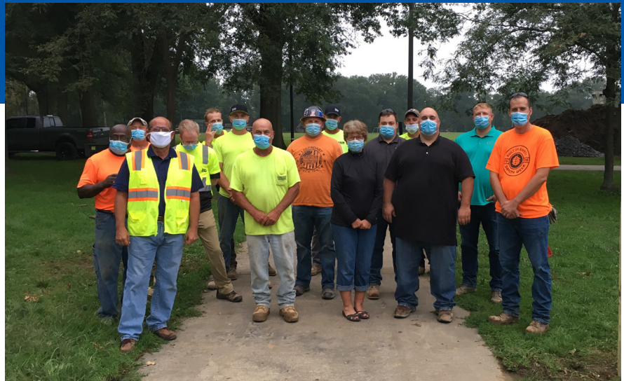
The team from Barton Malow, Jim Ledenko from Local 935 and Ginny Pasha break ground on the Born Learning Trail in Perkins Park.
